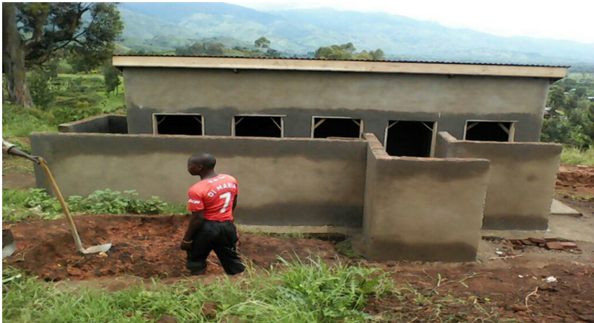
Figure 3.9 Example of in situ toilet/latrine construction by local mason: five stance lined pit latrine at Kisomoro Primary School, Uganda (Photo by Rutenta Allan, Source: https://rsr.akvo.org/fr/project/3890/update/19237 ).
