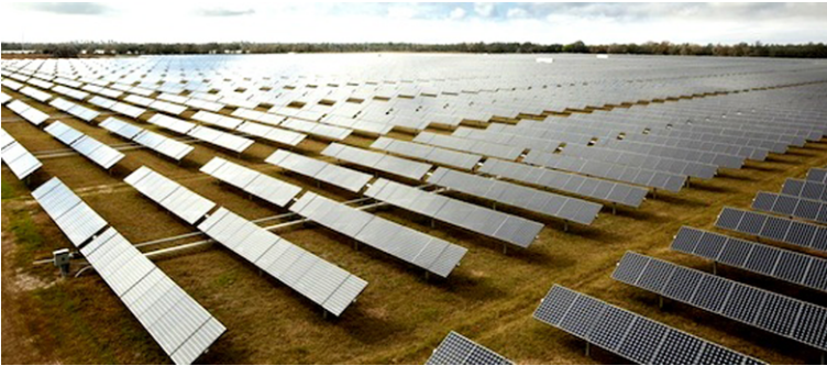
Figure 8.3 Ground-mounted PV (Source: NetZero Renewable Resources).
