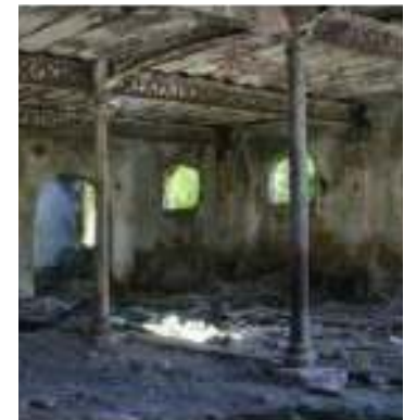
Fig. 8. Photograph of the state of the room with cast iron columns and beams in plot 2 (source: the authors).
