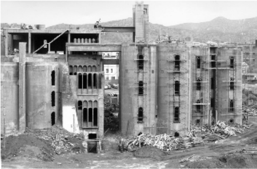
Fig. 8. Photograph showing the process of opening the windows in the cement silos, as well as the construction of the envelope (photo: Ricardo Bofill Archive).
