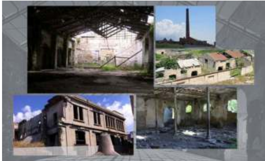
Fig. 4. State of some pavilions of the industrial complex of the former Corradini foundry in Naples (image: M. Falcone, G. Angrisani).
