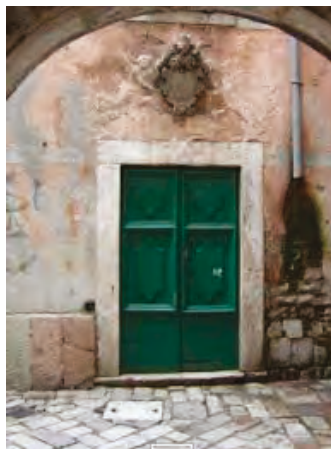
Figure 34. A door with no fanlights is framed with rectangular stone frames (Photo: Dušan Tomanović).
