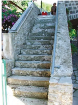
Figure 30. The tread and fence of the external stairway are mostly made of stone (Photo: Dušan Tomanović).
