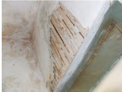
Figure 26. Dividing walls are made of wood and later plastered (Photo: Dušan Tomanović).
