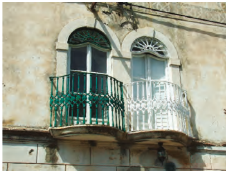
Figure 41. At the beginning of the 20th century, balcony fences were made from wrought iron (Photo: Dušan Tomanović).
