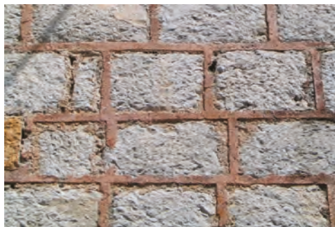
Figure 25. An example of a joint protruding out of the wall lines (Photo: Dušan Tomanović).
