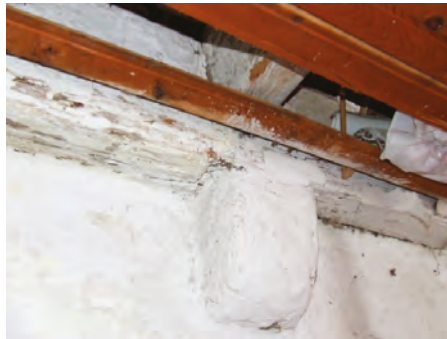
Figure 28. The small bracket carries the floor joist beam on the inner side of the wall (Photo: Dušan Tomanović).
