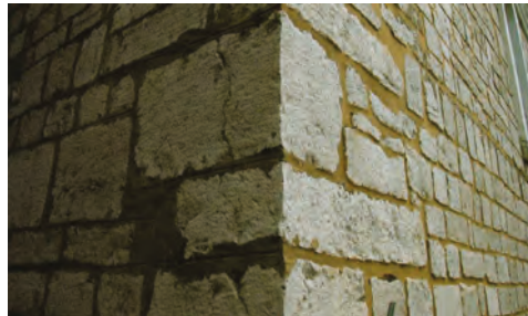
Figure 23. The corners of the house were made using blocks of greater length (Photo: Dušan Tomanović).
