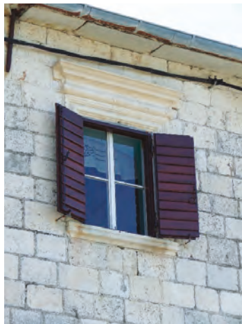
Figure 33. Windows on multiple-storey houses were defined by the quality of the window frame (Photo: Dušan Tomanović).
