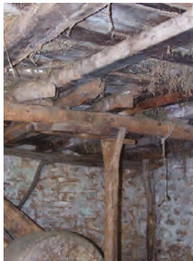
Figure 21. Roof construction is supported by a wooden forked pole (Photo: Dušan Tomanović).
