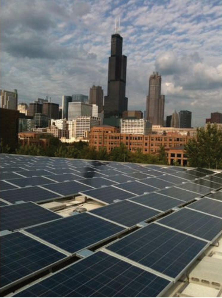
Figure 4. Rooftop Solar Installations Rooftop solar installation on Douglas Hall at the University of Illinois at Chicago has no effect on land resources, while producing electricity with zero emissions. Source: Office of Sustainability, UIC
