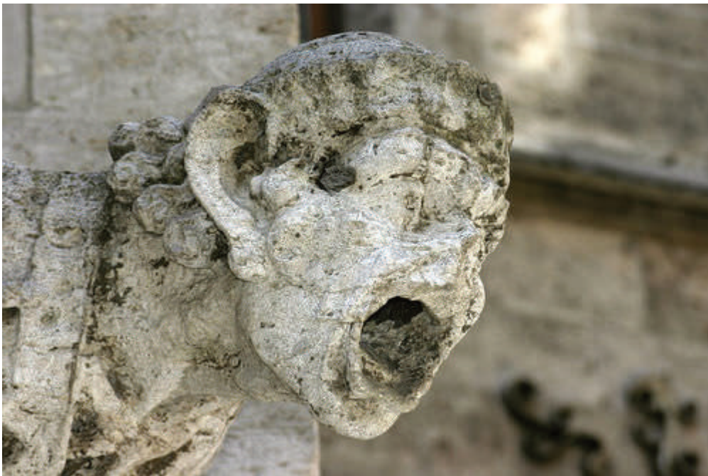
Figure 2. A gargoyle that has been damaged by acid rain.
